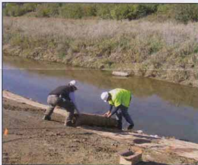
Erosion control matting being spread along the south bank of Dicks Creek during the phytoremediation work.
